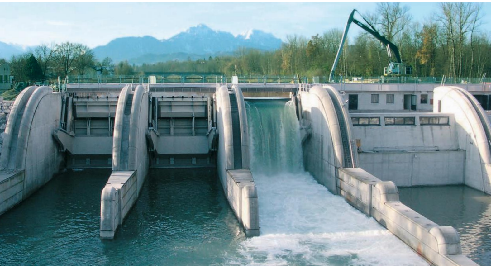
The weir with the three gates, of which each gate has a clear width of 9 meters.
