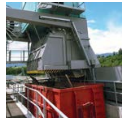
Intermediate storage and container
